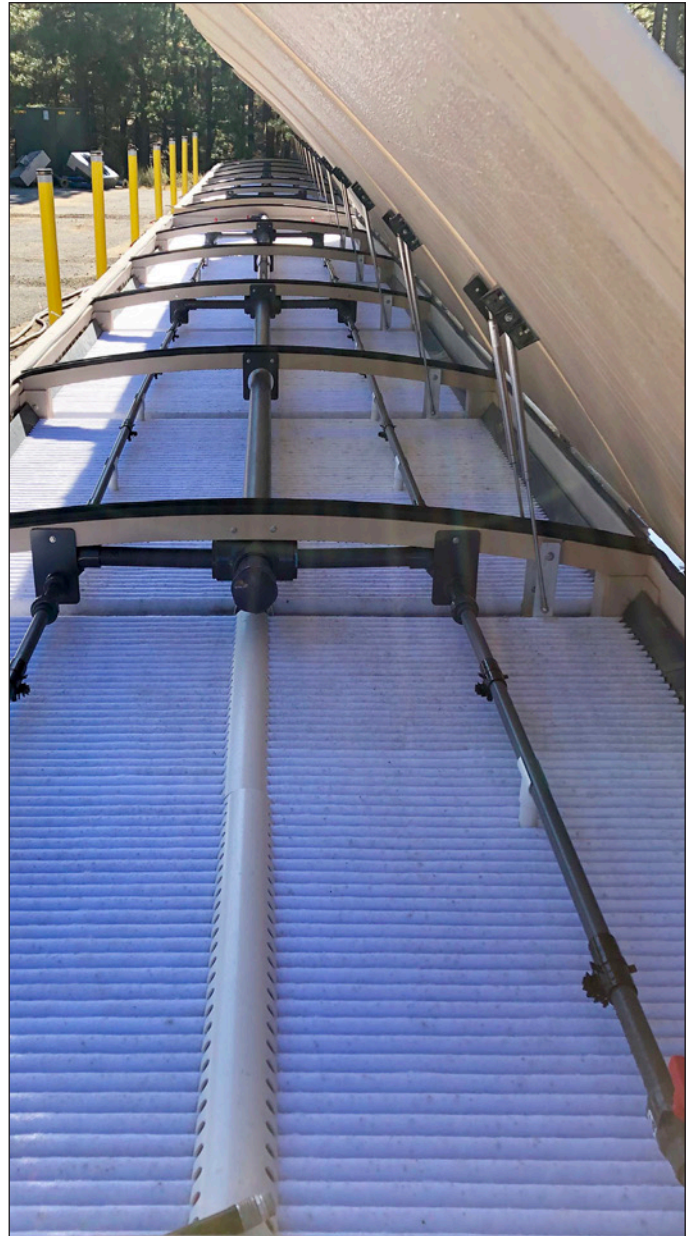
An AdvanTex® Treatment System was chosen because it can handle low and inconsistent flows and be put into operation soon after installation.
